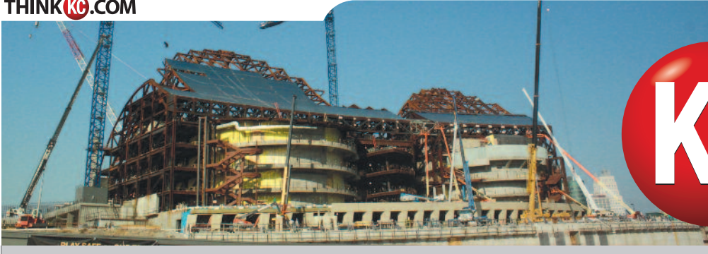
The Kauffman Center for the Performing Arts begins to take shape in downtown Kansas City, Mo.
